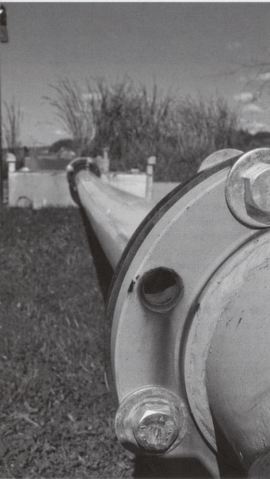
The water pipe system pumping into Lake Mendota stationed along Lakeshore path
