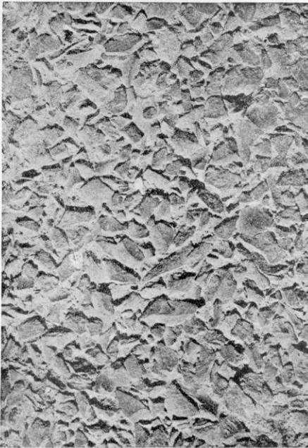
CONCRETE, COMPOSED OF ONE PART CEMENT, TWO PARTS YELLOW BANK SAND, AND THREE PARTS THREE-EIGHTHS-INCH SCREENED STONE
