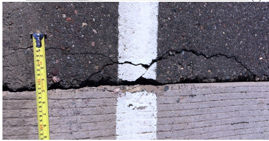
Figure 3.9. (a) Crack observed in May of 2013 at the edge between the deck (bottom) and approaching road (top) at the south-east end. (b) New crack observed in March 2014 right next to the old one.
