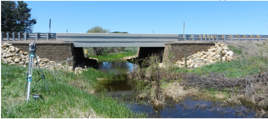
Figure 4.2. (a) Location of the GRS-IBS bridge. The red circle indicates the location of the bridge. (b) Picture of the GRS-IBS bridge.
