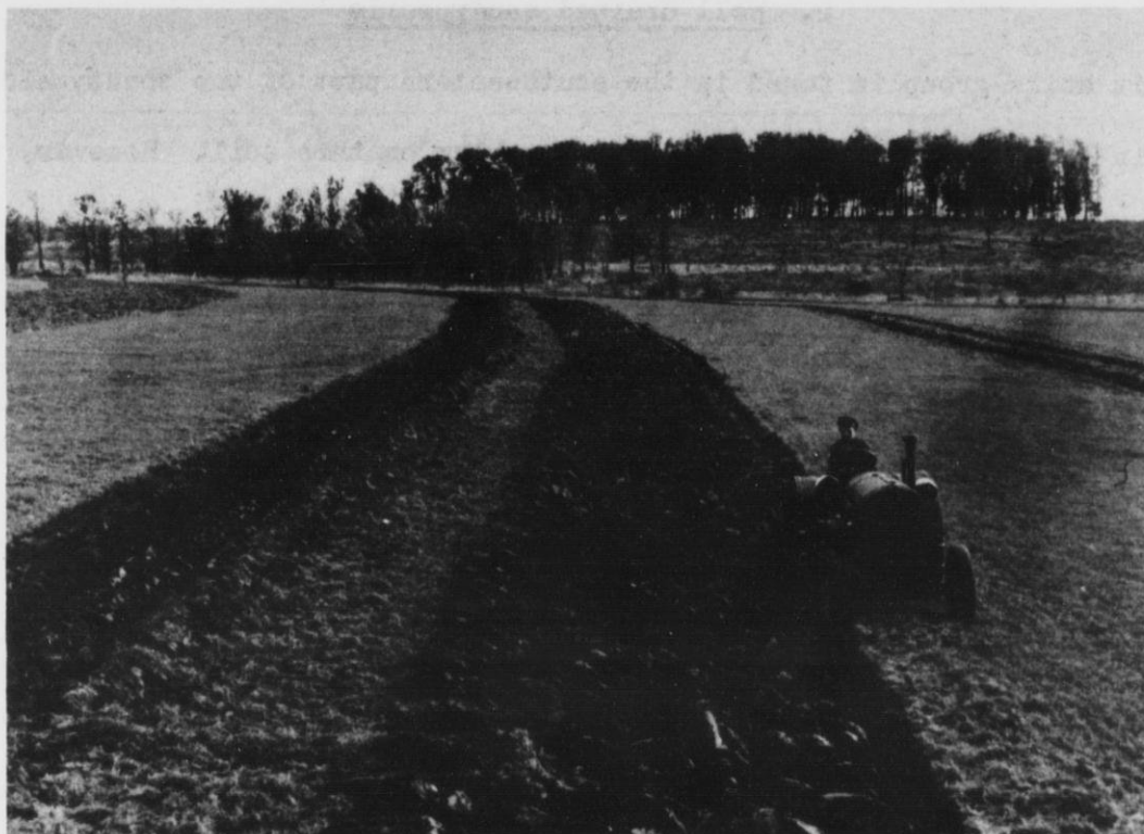
Erosion control and water disposal terrace being constructed using Island method - Edgar Lubeck farm, Arpin township.
