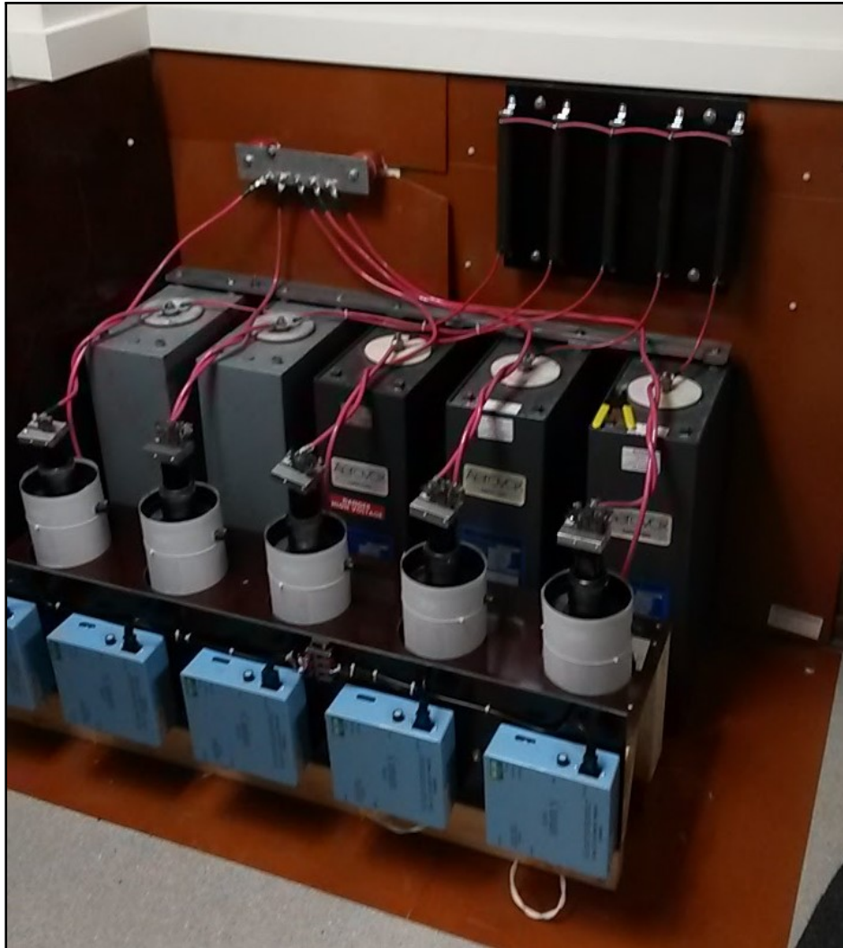
Figure 3.5: A picture of the 5 capacitor heater drive circuit. Each branch consists of a capacitor with its own high voltage ignitron switch. The blue boxes are Northstar IG5F2 drivers for triggering each ignitron.
