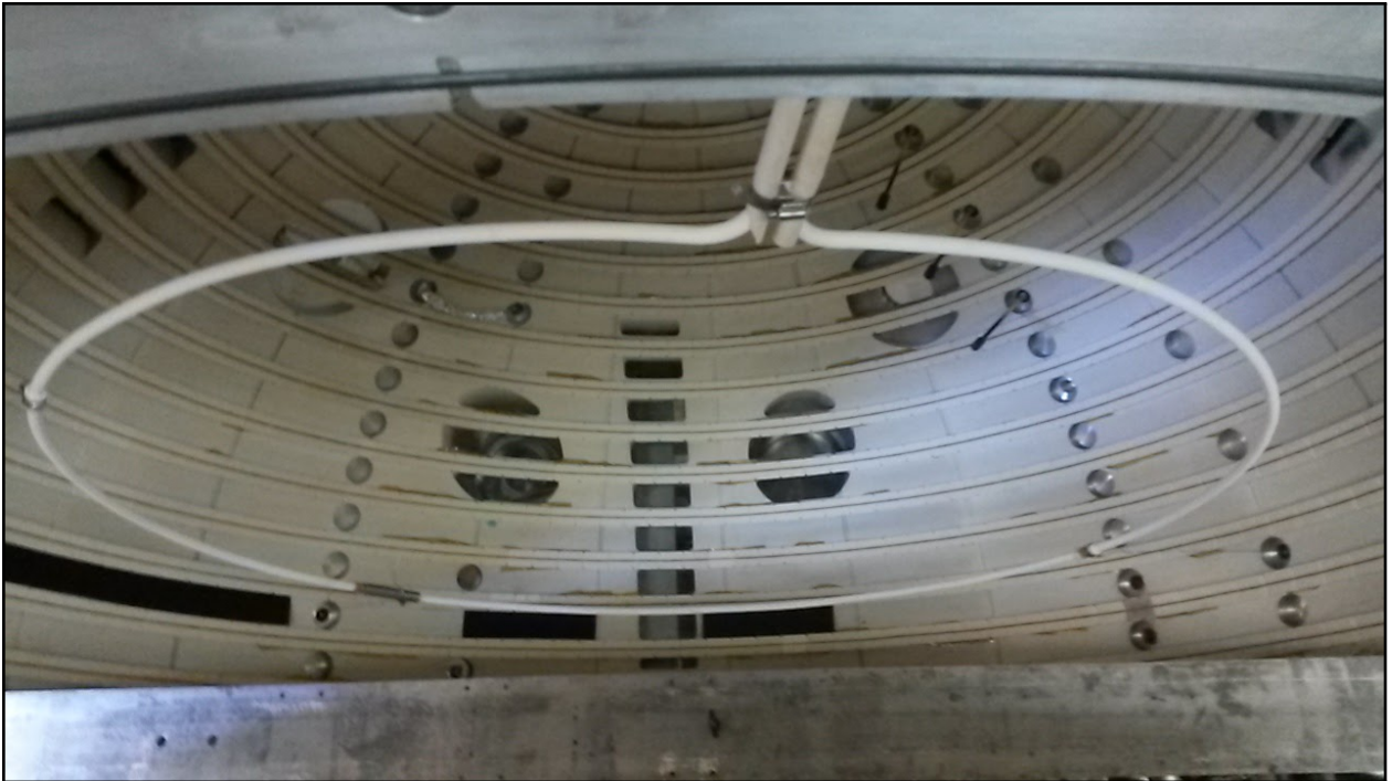
Figure 3.1: A single internal drive coil inside the BRB vessel during installation and alignment.
