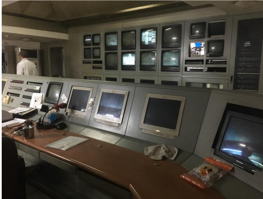
(The surveillance and control center)
