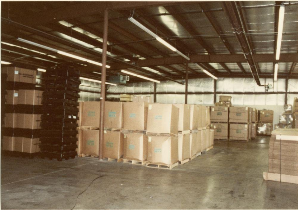
Interior of east section of warehouse occupied by Kippcast. Note ceiling and wall insulation, piping for sprinklers and fluorescent lighting. Space heater at upper left.
