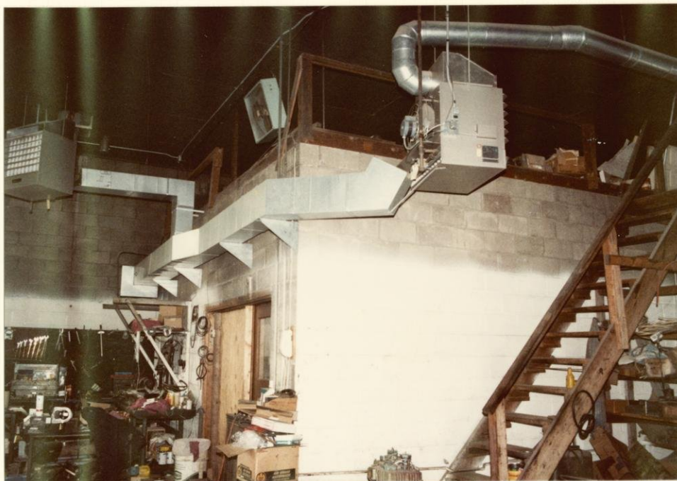
Interior of 2957 Packers Avenue. Note concrete block exterior wall of office with storage above. Also note newly installed gas space heaters.
