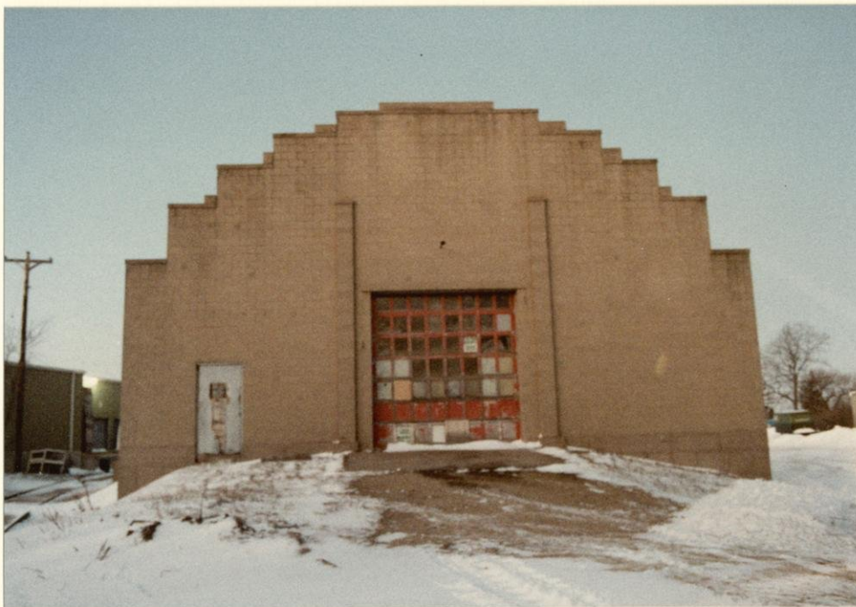
Concrete block endwall at east end of quonset warehouse at 2955 Packers Avenue. Note rail spur on south side of building.
