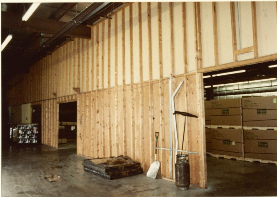
Plywood wind barrier to protect main warehouse storage area from dock area. Plywood shields have been installed in both sections of the building parallel to the dock area.
