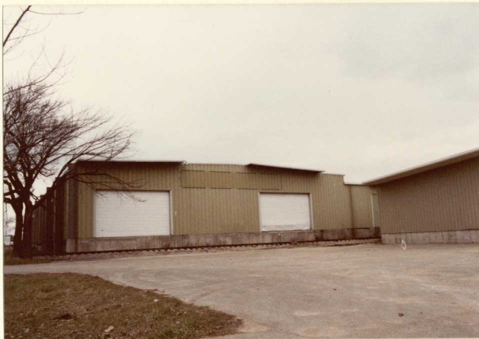
Rail dock doors on south side of 625 Mayfair Avenue. Rail spur runs parallel to building.
