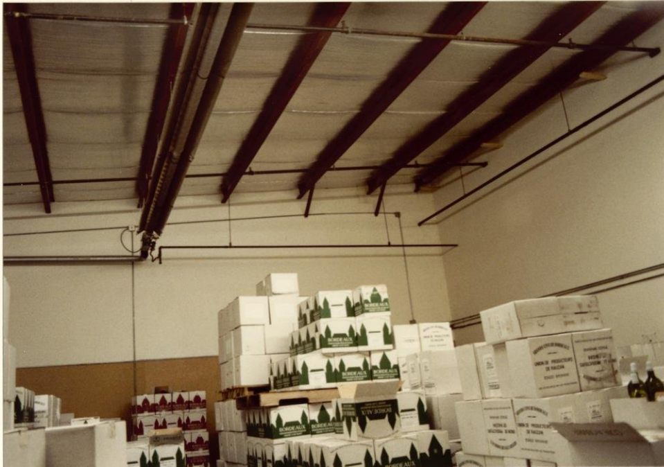
Interior of Amboise Cellars' space at 2201 Darwin Road. Note interior finish, sprinklers and lighting.
