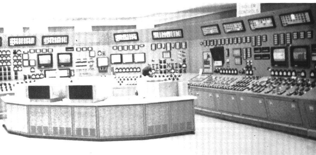
The control center of the Columbia II Nuclear Power Plant, Wisconsin
