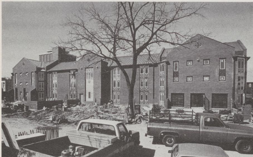
Merit House, at Dayton and Park streets, in late-April stages of completion.
