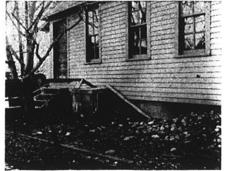
Air intake to a basement storage where the air duct is built on the outside. Such openings should be fitted with airtight doors and be located about fifteen feet apart on the sides and ends of the house.
