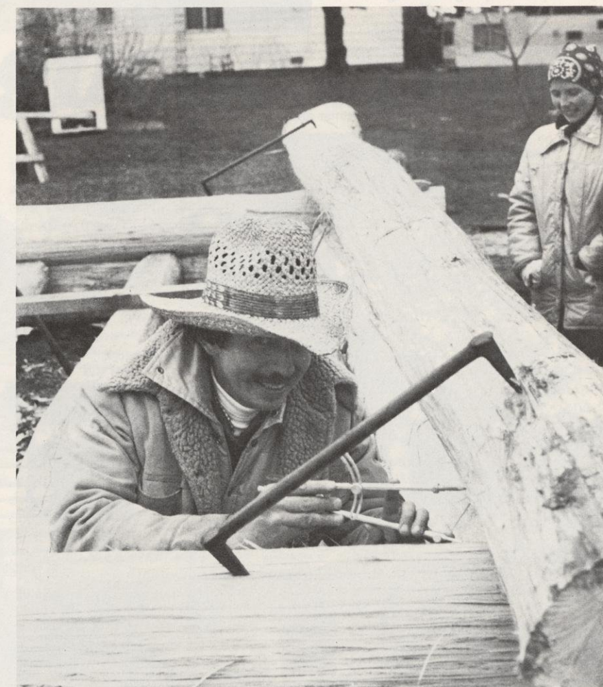
"Log dogs" hold a log in place while Palmquist marks a notch with a compass. This large compass with a two-way level helps ensure accurate markings since "the trick is to keep the point exactly plumb or perpendicular." Photo by Cedric Vig
