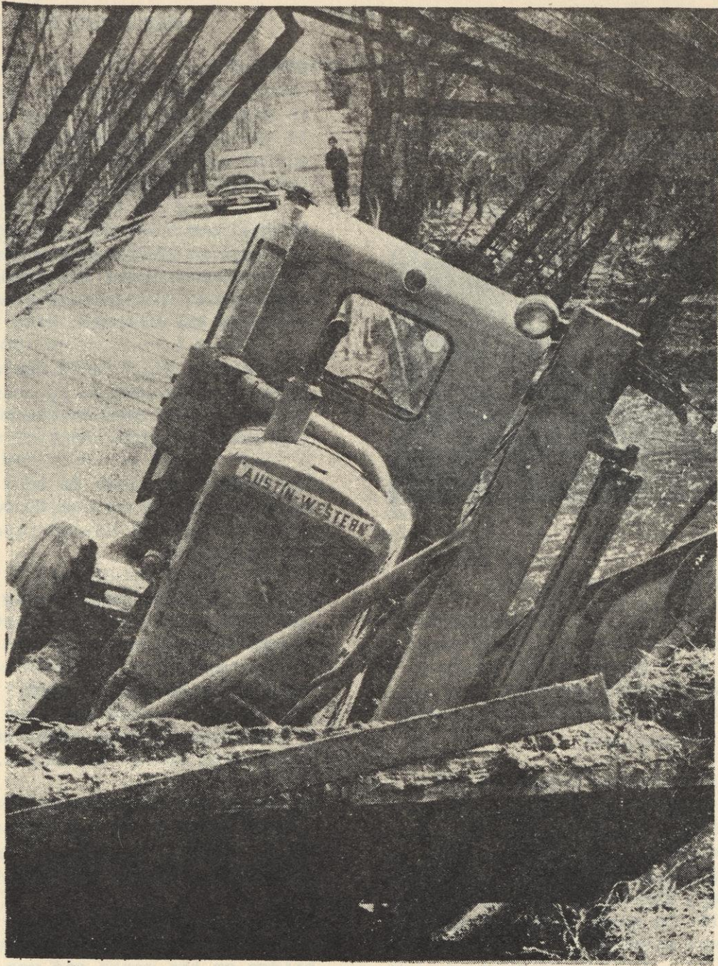
... Record-Herald Photo TEN-TON ROAD GRADER WAS STRAW THAT BROKE BRIDGE'S BACK Town of Texas Bridge Gives Way After 48 Years of Service
