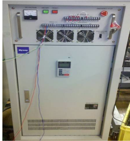
Fig. 2.26 MYWAY Inverter for FI-IPMSM and YASAKAWA drive (bottom) for induction machine
