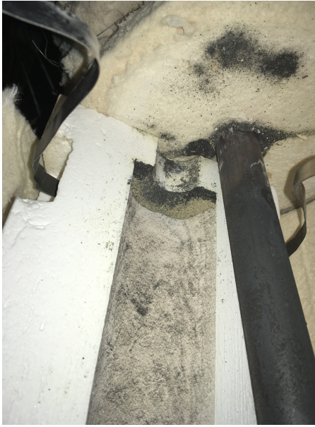
Figure C.8: Stainless oxide collecting at the bottom of heater 3 along the riser.
