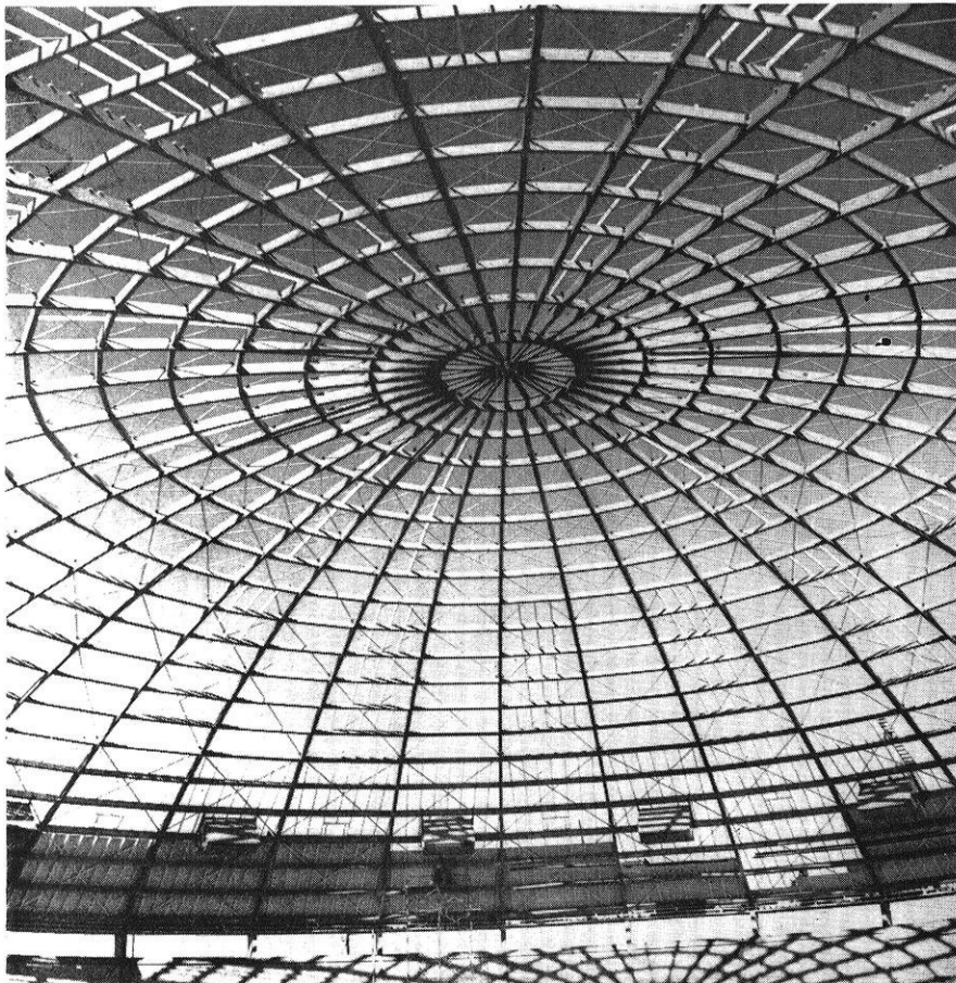
Timbers of glued laminated Douglas fir presented a dramatic pattern of structure and shadow as Timber Structures, Inc., roofed this building in time for the 1957 basketball season. It's the main arena of Montana State College's new physical education center at Bozeman, Mont. World's widest span timber structure, the arena is 300 feet in diameter. Giant wood arches rise to 90 feet at center.
