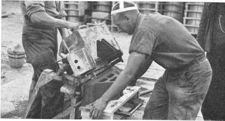
To reduce costs, pre-cast concrete blocks are made at many of the building sites.
