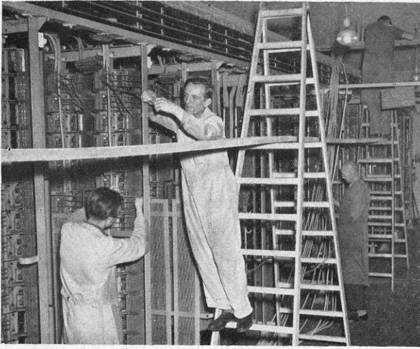
Workmen repairing one of the nine telephone exchanges in the U.S. Sector damaged by war-time bombing.
