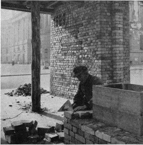
Repair work often had to start from the ground up. Germany's Lebensraum problem—a Nazi excuse for aggression—was somewhat intensified during the war.
