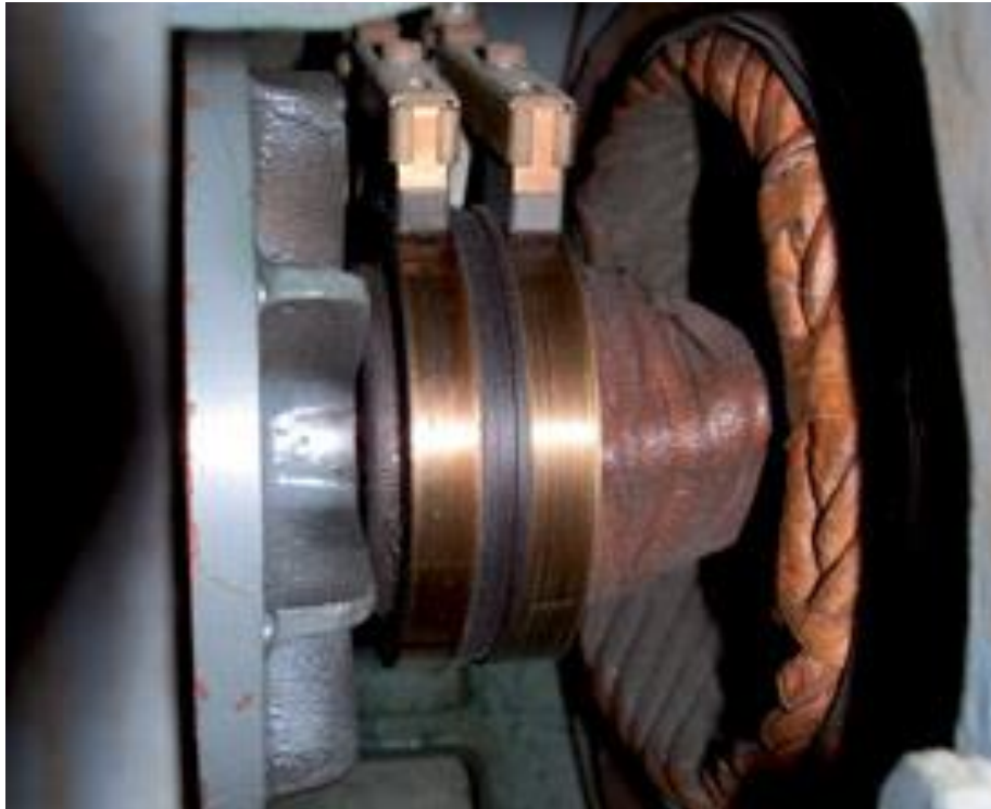
Figure 1-1: Photograph of carbon brushes sliding on rotating slip rings. [5]
