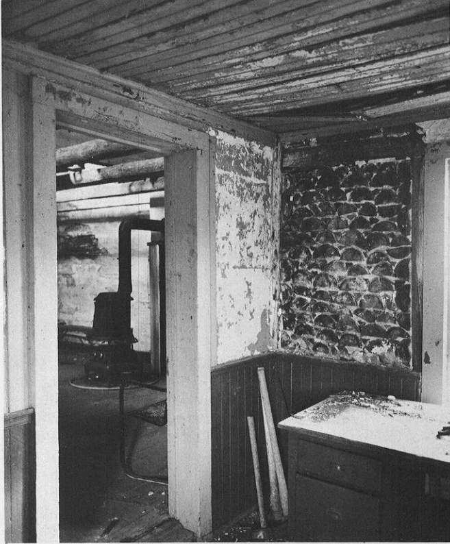
A common situation was the use of stovewood for an addition to an existing log or stone house. This kitchen wing was added to the William Zachow residence near Ephraim in 1909-10.
