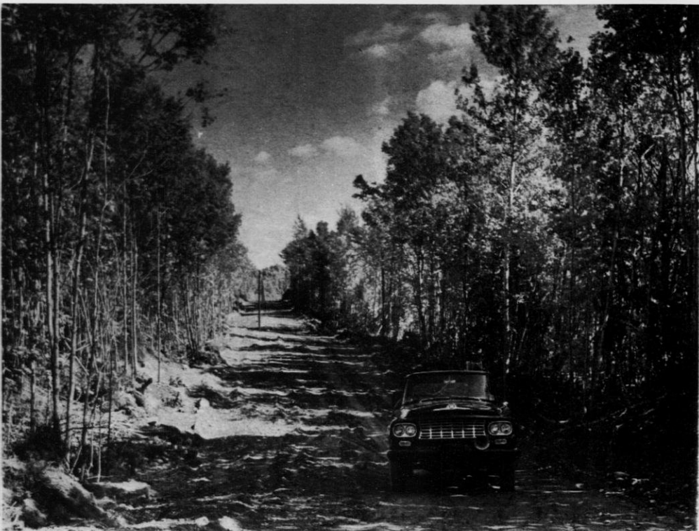
A new telephone line and road in Iron county were made possible by Economic Opportunity Act funds.
