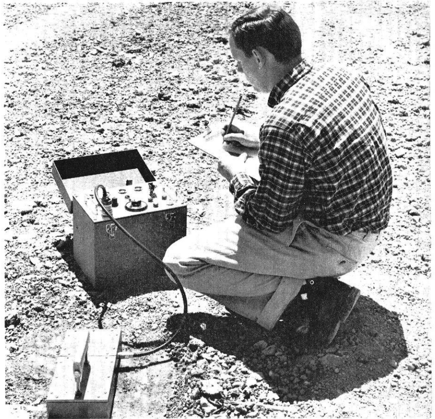
Operator obtains final surface density (or surface moisture) reading on the construction site. Total time elapsed for entire operation: three minutes.
