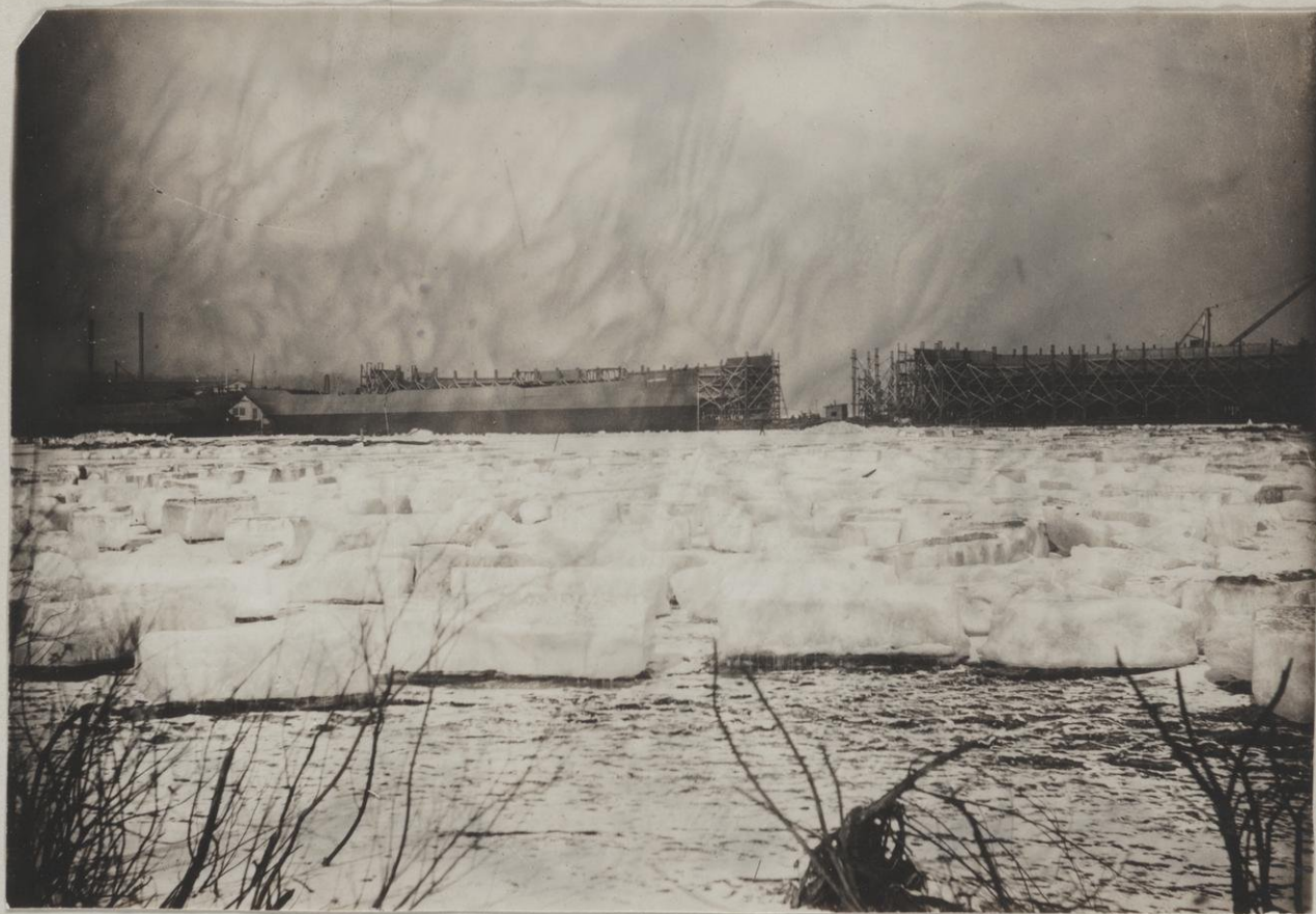
From November 8th, 1917 to February 20, 1918, we built four ships while the ice formed 38 inches thick. We cut and pulled out 6000 tons of this ice to launch the first of these ships. During this time, we increased our plant to a ten-berth shipyard.
