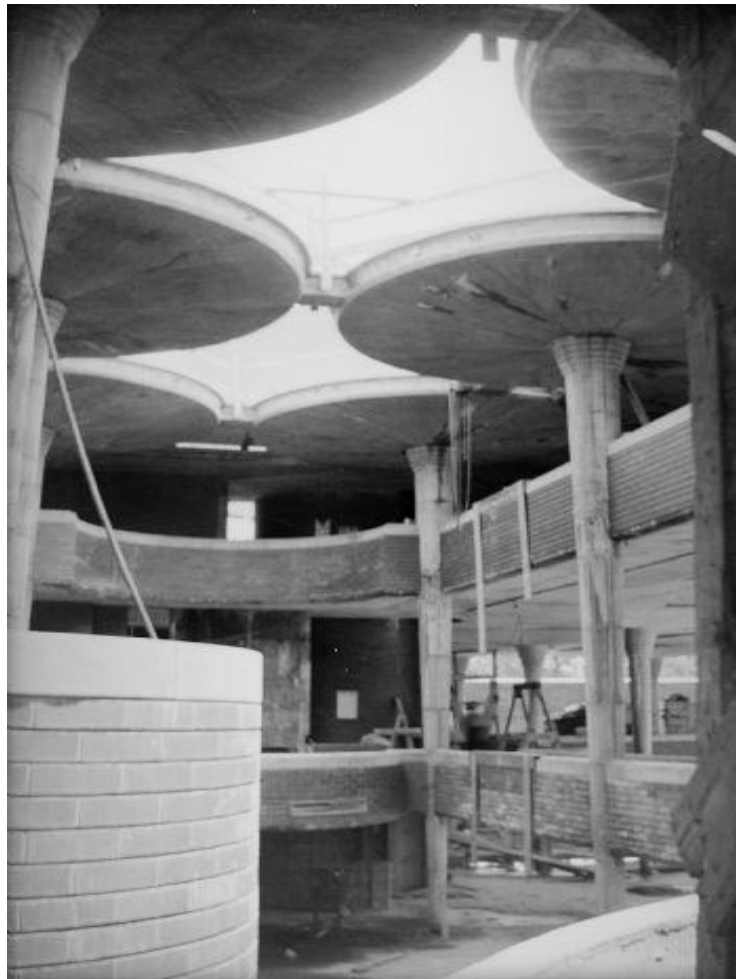
Figure 36. The Great Workroom under construction. Wright pushed available construction technology to its limits to flood the Great Workroom with light. The effect was intended to parallel an experience in a cathedral (Courtesy the Historical Society of Wisconsin, John Howe, ca. 1936).
