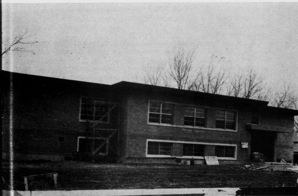
Here is the new Oshkosh conservation area headquarters under construction. The building was completed and occupied in 1956.
