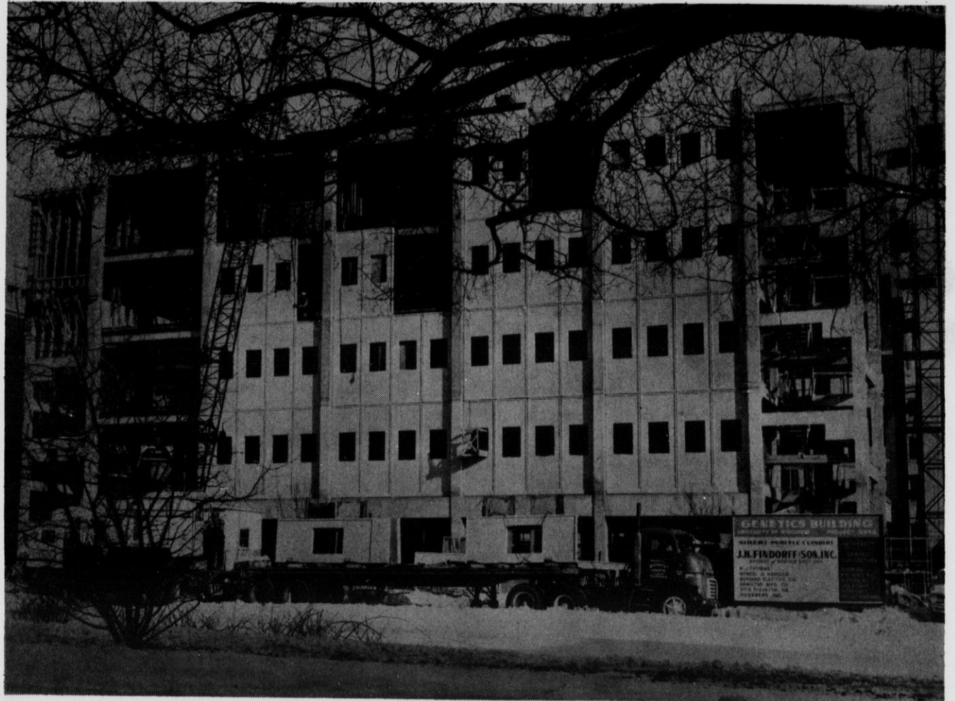
Construction of the new Genetics Building, directly across from the old building. January 1962
