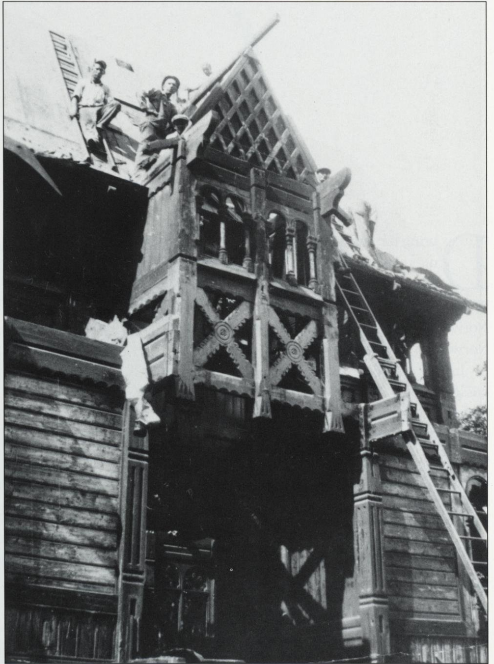
The building's construction elements are very visible in this photo taken during its dismantling at Lake Geneva. Little Norway Collection.
