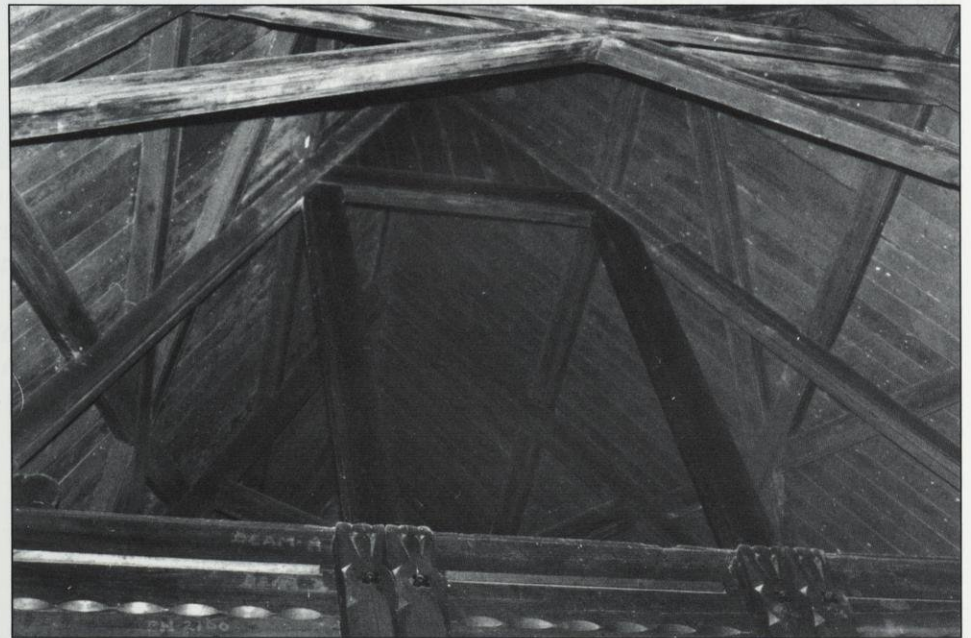
The Norway Building's roof construction includes scissor-bracing (top) and nave posts, connecting the roof to the staves (below). Photo by Randy Winner. Little Norway Collection.
