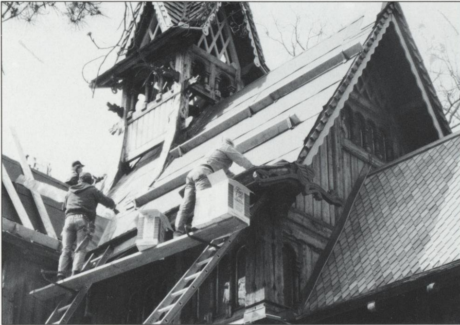
Workers prepare the roof of the Norway Building for custom-made dragon-scale shingles during restoration of the building in the Spring of 1992. Little Norway Collection.
