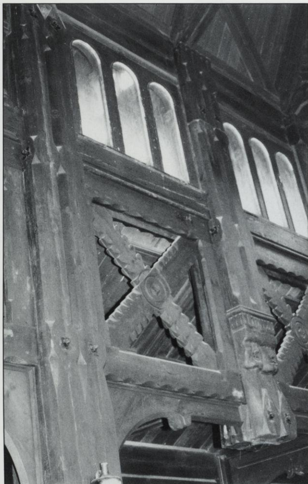
Upper detail of the Norway Building's nave shows the clerestory windows and St. Andrew's crosses.
