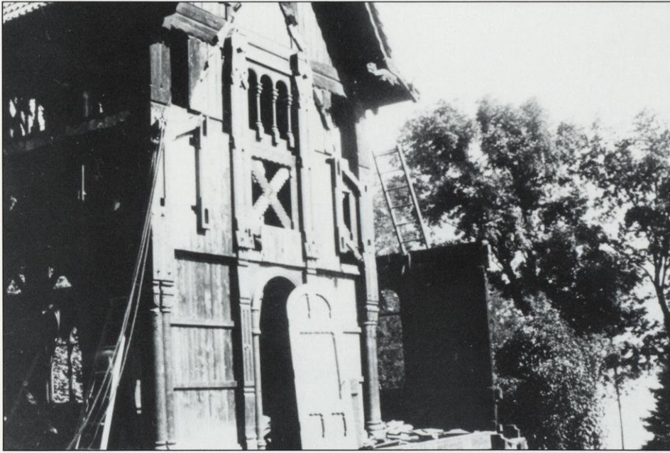
The door, which has been removed from its hinges, served as the entrance to the Commissioner's office during the Fair. Dismantling, Lake Geneva, 1935.
