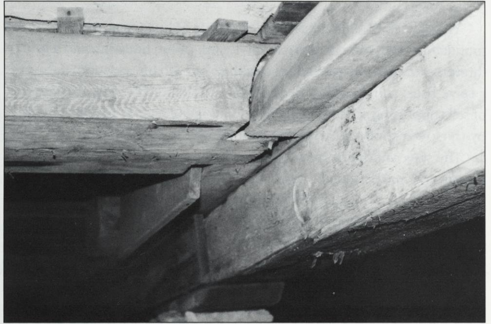
The Norway Building's chassis is evident in this photo, taken beneath the building. Little Norway Collection.
