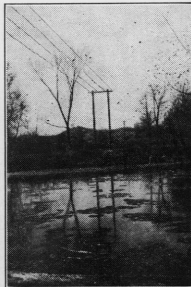
Three phase river crossing. Trempealeau project.
