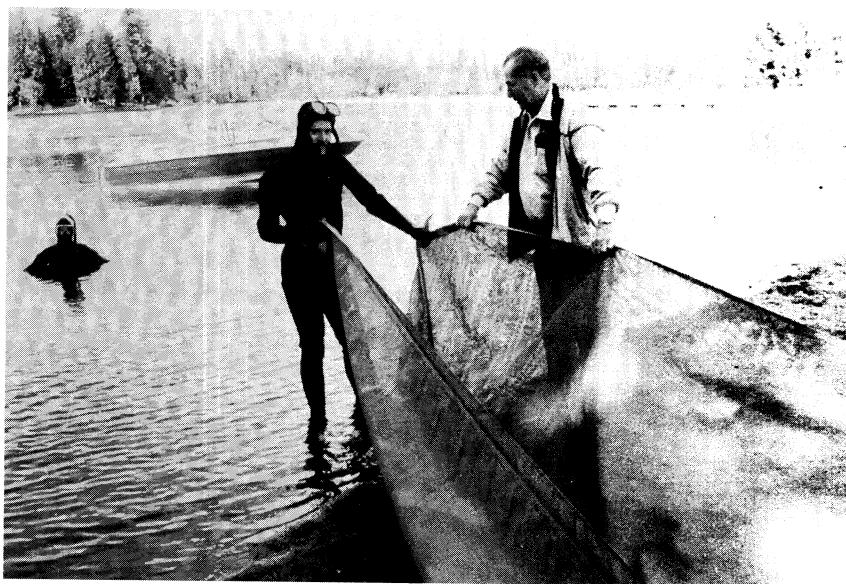
A fiberglass screen, weighted with rebar, being set by divers on the bottom of Pipe Lake, King County, Washington.
