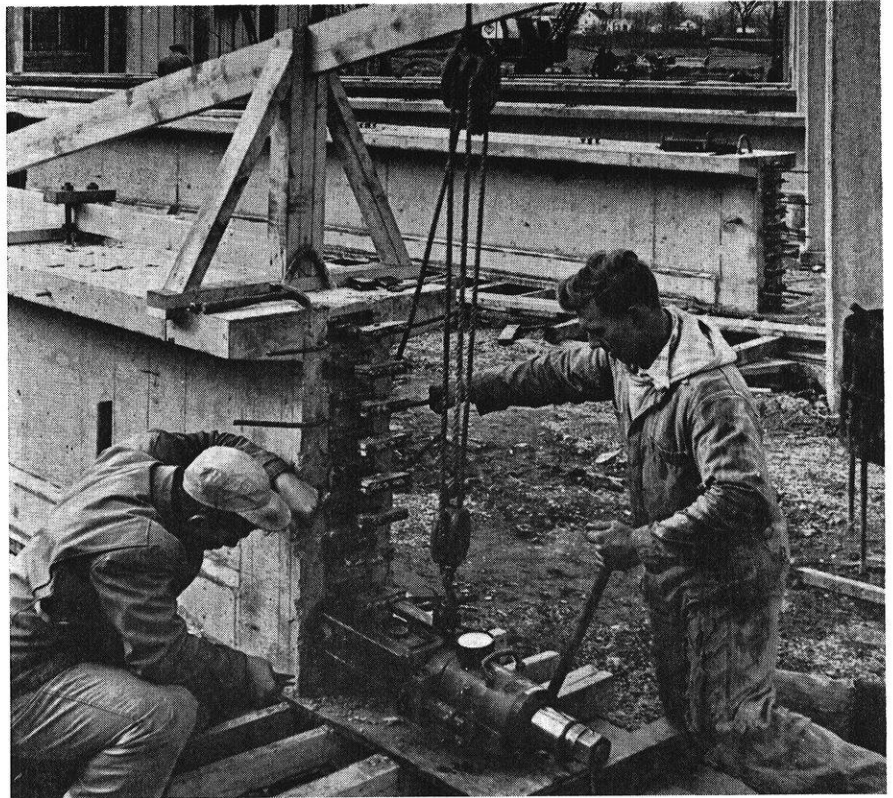
This photograph shows how the reinforcing steel is tensioned by a hydraulic jack to produce prestressed concrete beams.
