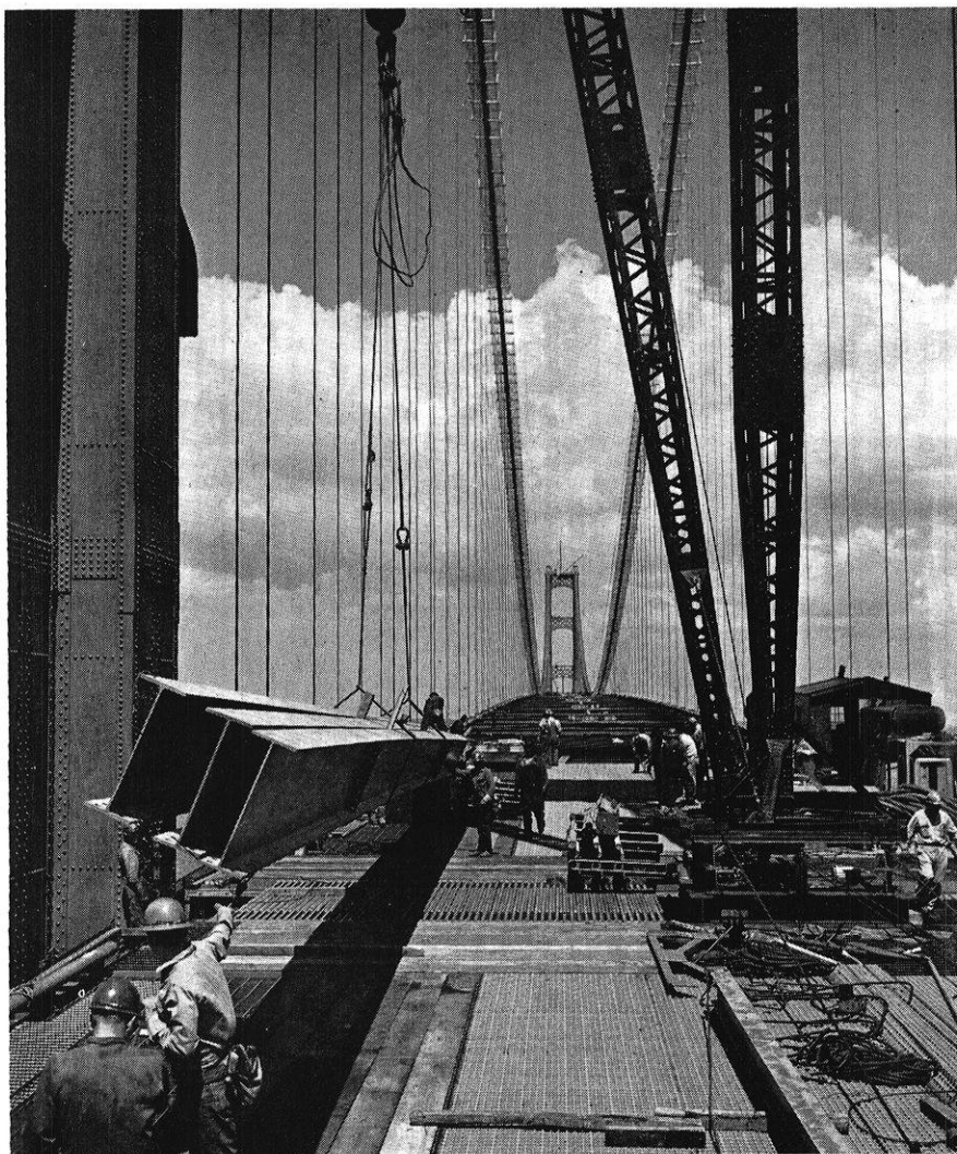
Roadway stringers are lifted from the barge to the roadway for the suspended span of the bridge. These are moved by temporary derricks such as the one set up at the right.
