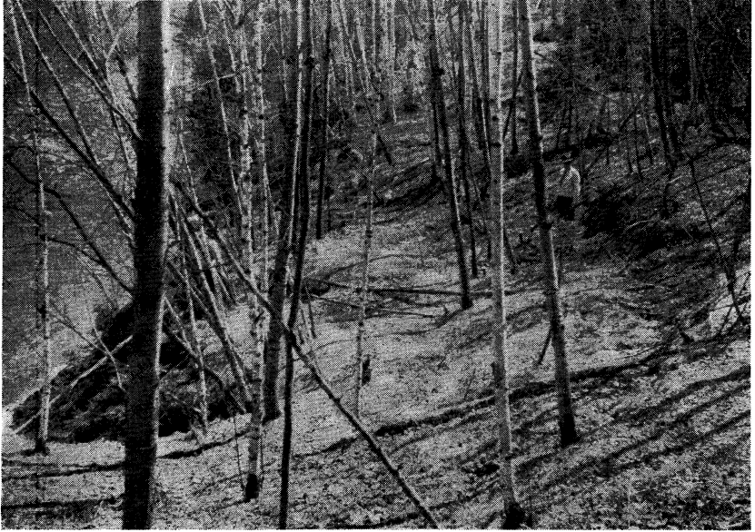
PLATE 11. Section of slumping bank below N. P. Johnson Bridge showing large mass moving down into stream. Recent drop of more than a foot showed along the line where the man is standing.
