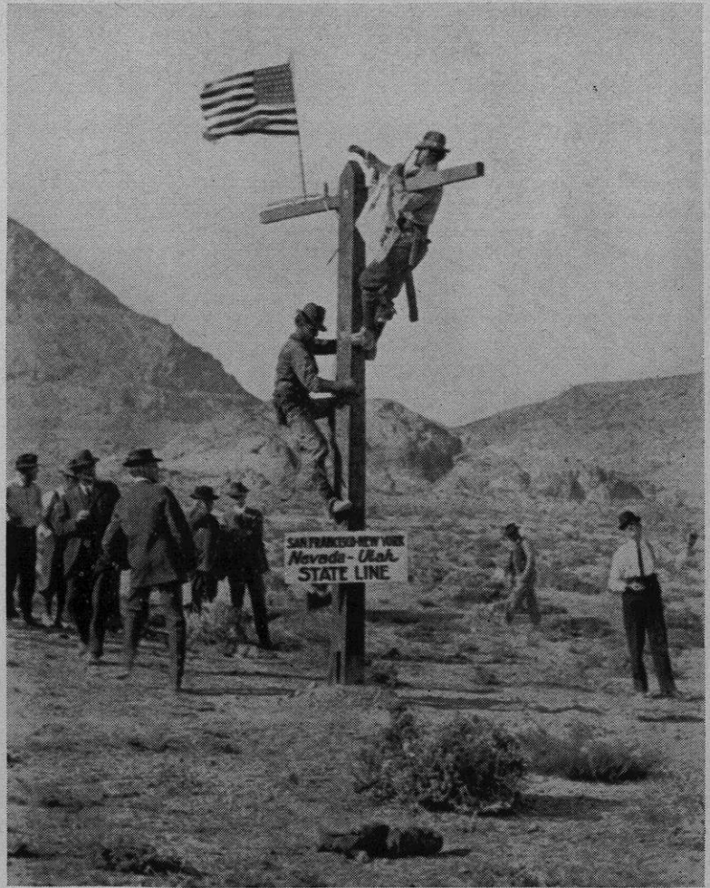
The first open wire line (linked here at the Nevada-Utah border) could carry only three calls and was vulnerable to interruptions.
