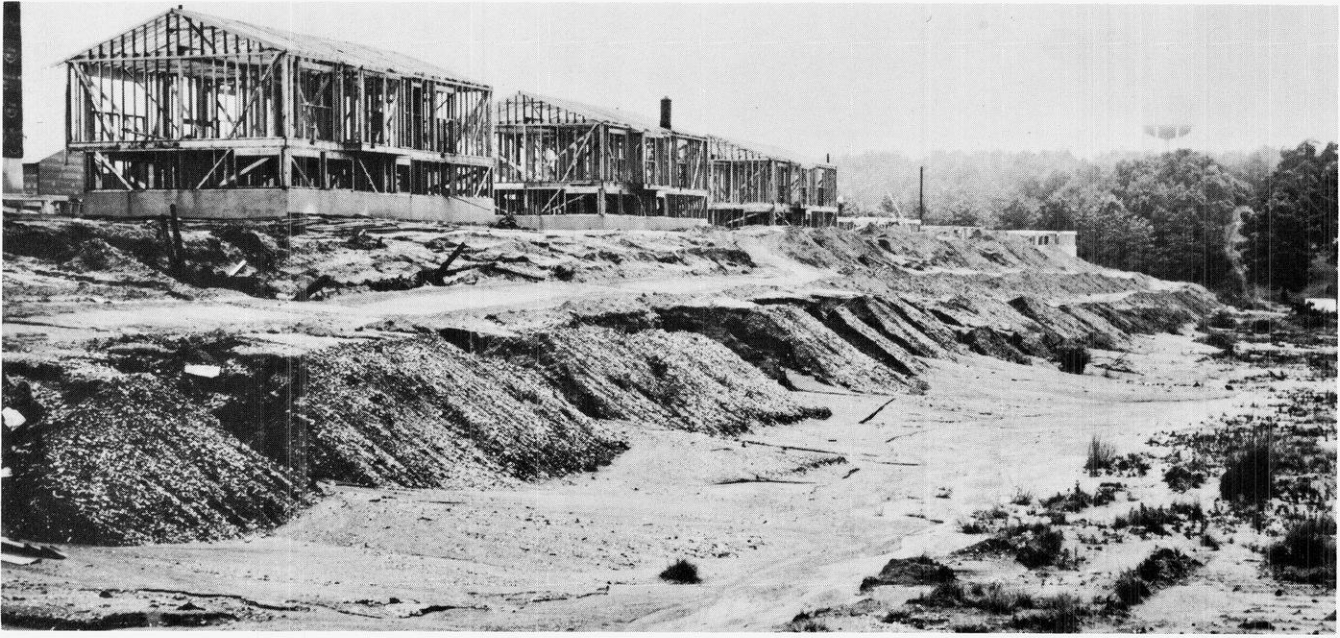
Figure 20 POOR PRIVATE DEVELOPMENT PRACTICES
