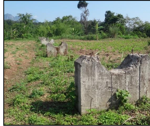
Figure 4.10: Remnant pipe holders left from failed government water pipe project. Photograph by P. Vue.
