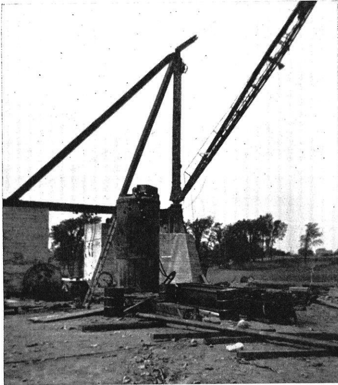
Fig. 2. Stiff-Leg Derrick Mounted on Sunken Concrete Blocks. Note Core Barrel in Foreground
