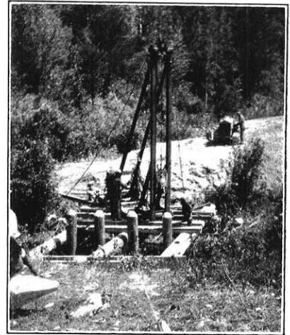
Driving Piling for a 25-ft. Bridge with a Renovated Abandoned County Pile Driver.
