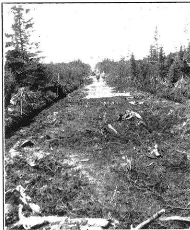
Five Hundred Feet of Corduroy Required on Either Side of a 15-ft. Bridge Crossing.
