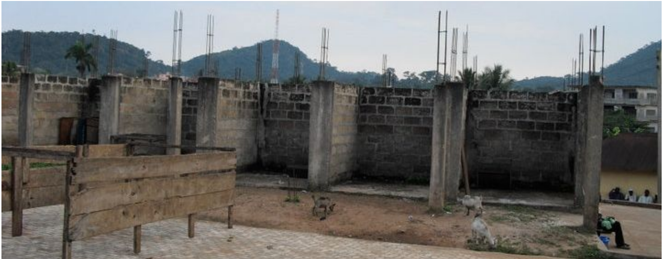
FIGURE 5.6: Unfinished market stalls, three years after construction began
