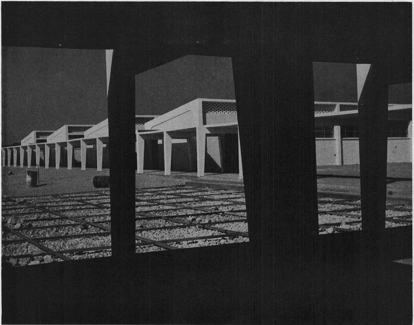
The New—This ultra-modern architecture marks the home of the Gaza Vocational Training Center. It is supported by UNRWA and the Egyptian government.
