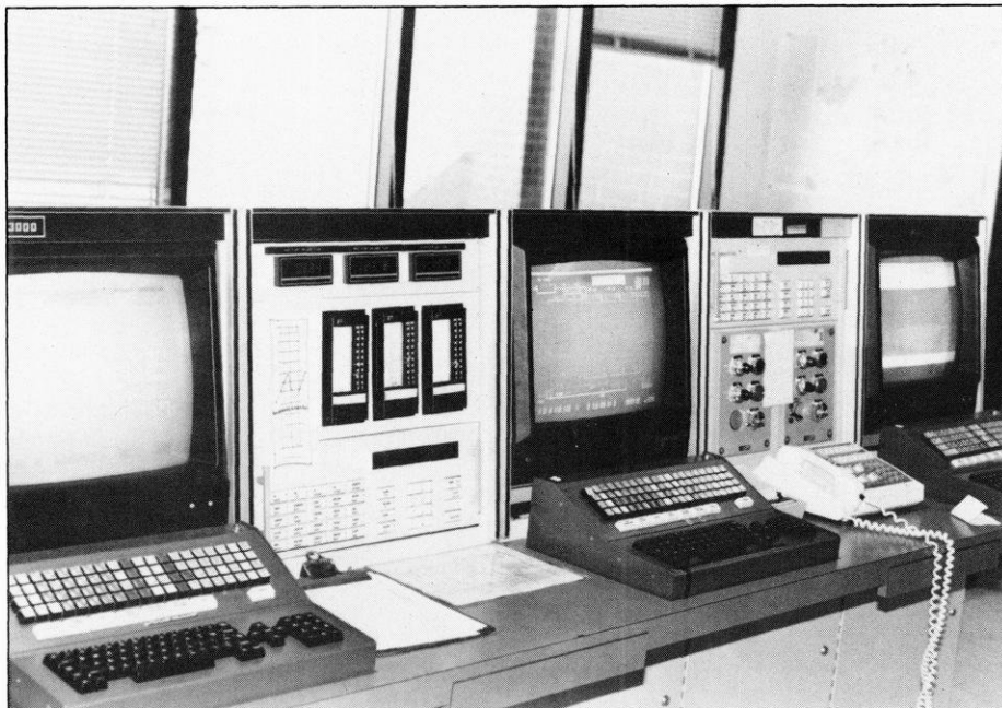
Multiple gauges and screens show results of continuous monitoring of the many processes of the sewage treatment plant. Keyboards allow plant operators to adjust parameters, if needed.
