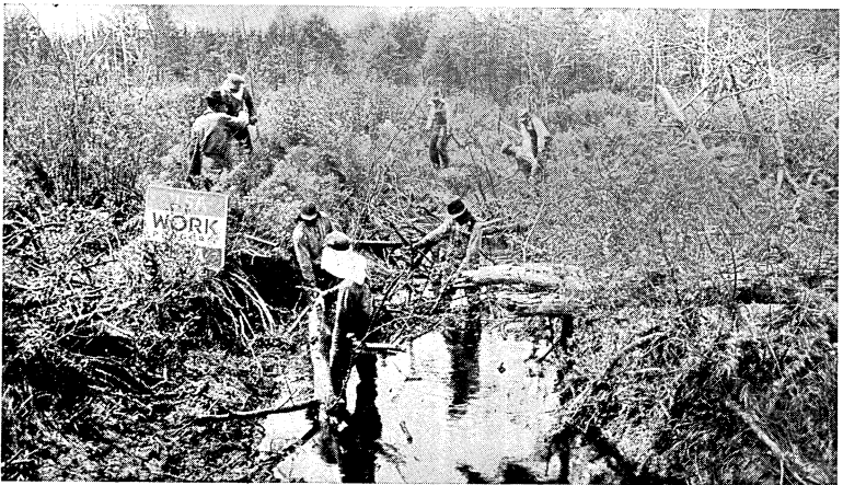
Stream improvement. WPA workers clear streams of underbrush so there will be a better flow and a good place for trout.
