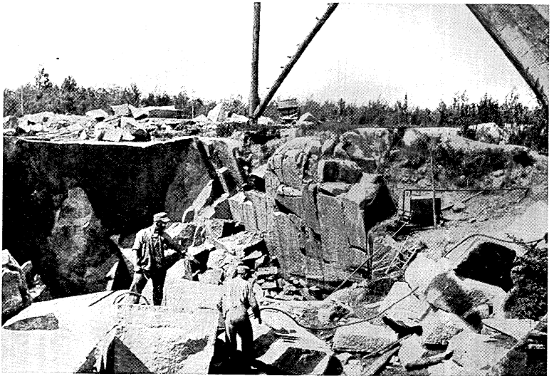
The Amberg Quarry operated by the State Reformatory where granite is being quarried and prepared for the new state office building.
