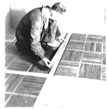
FIG. 7—Laying a hardwood floor. T-shaped hardwood strips hold the prefabricated squares solidly to the panel subfloor.
