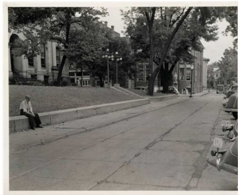
Figure 3.3: Photograph of oldest concrete street in America, Ohio State Archives, State Archives Series 741 AV, Box 3, Folder 43, Ohio History Connection. Accessed June 2019 at https://ohiomemory.org/digital/collection/p267401coll32/id/14423/ .
