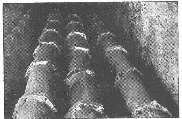
Section of 285-year-old cast iron water main still serving the town and fountains of Versailles, France.
