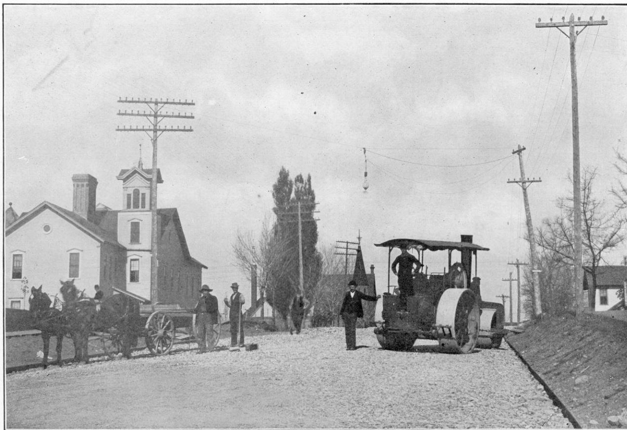
A Macadam Pavement with Plank Curb, Showing the Usual Style of Steam Roller.
