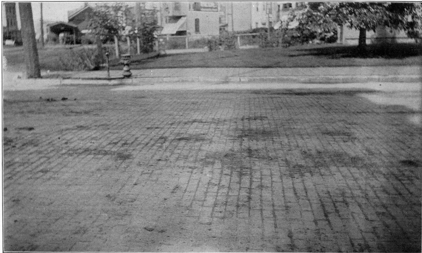
Brick Pavement Cement Grouting Filling Joints. Algoma Street, between Main Street and the Wisconsin Central Railway Tracks, Oshkosh, Wis.
