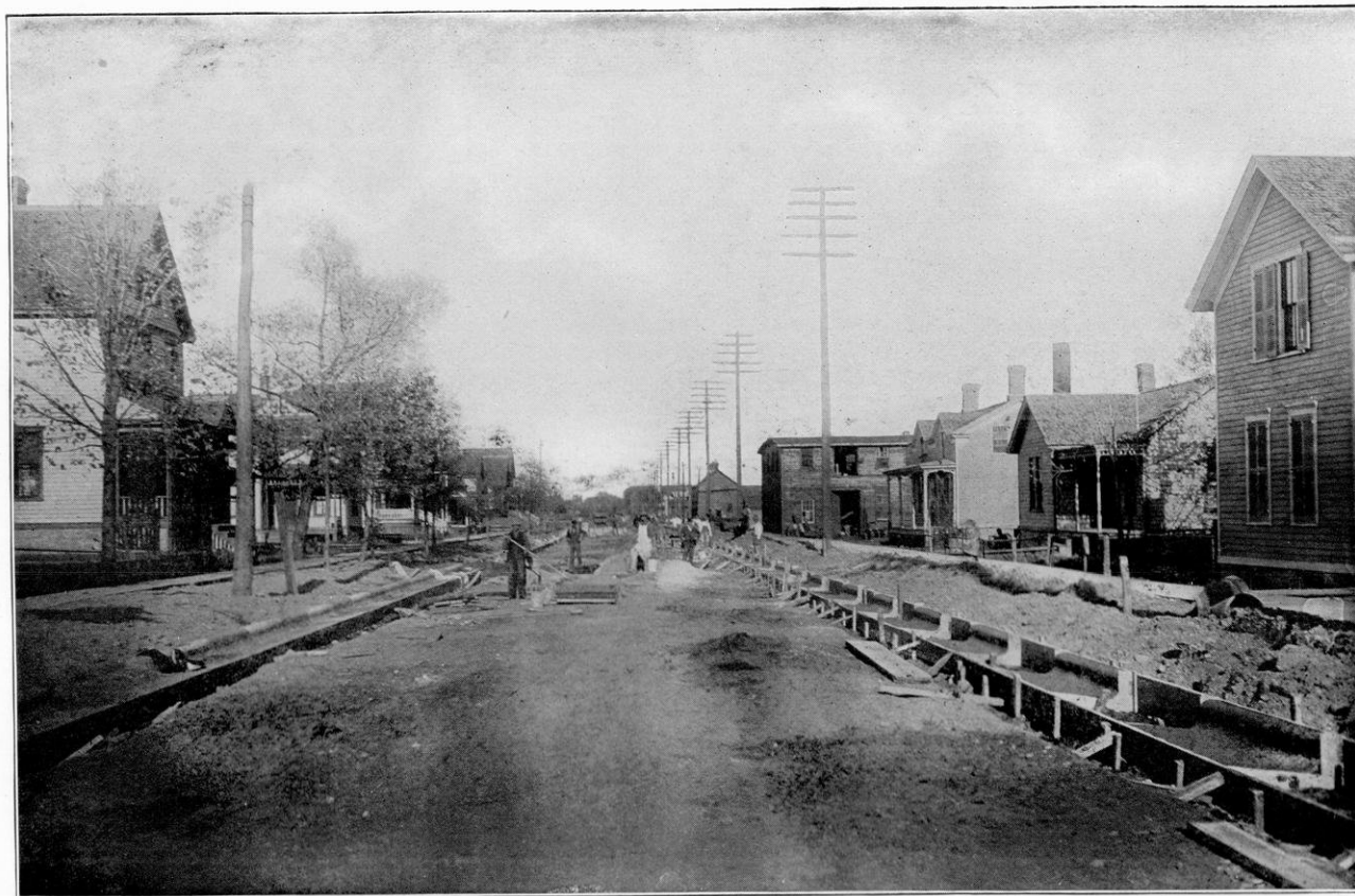
Constructing Combined Cement Curb and Gutter before Laying Macadam, East Mifflin Street, Madison, Wis.
