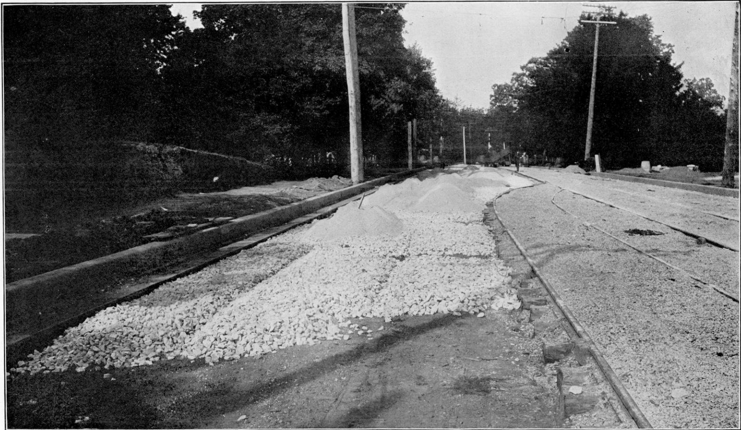
Macadam Pavement in Process of Construction, Showing Combined Cement Curb and Gutter, Washington Avenue, Racine, Wis.
