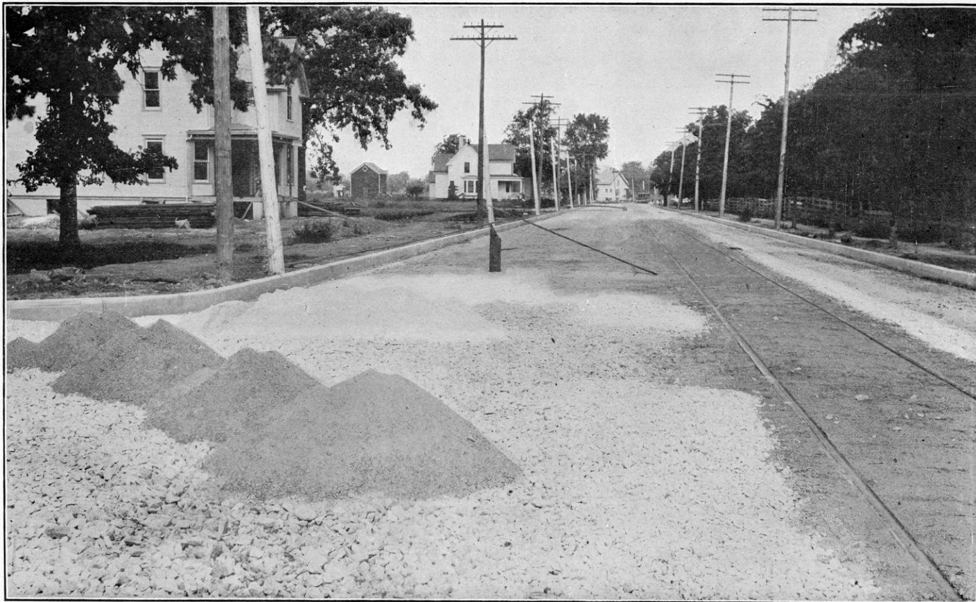
Macadam Pavement in Process of Construction. Washington Avenue, Racine, Wis. Top dressing in piles in foreground. Finished street in the distance.
