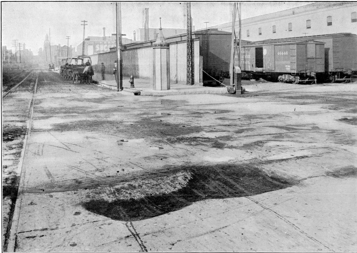
Asphalt Pavement. Intersection of Chestnut and Third Streets, Milwaukee, Wis. Shows the effect of heavy traffic.
