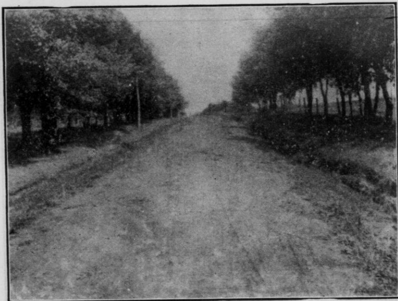
A good piece of earth road in the Town of Christiana, Dane Co. Graded with traction engine and kept in shape with road drag. This town has many miles of such roads.
