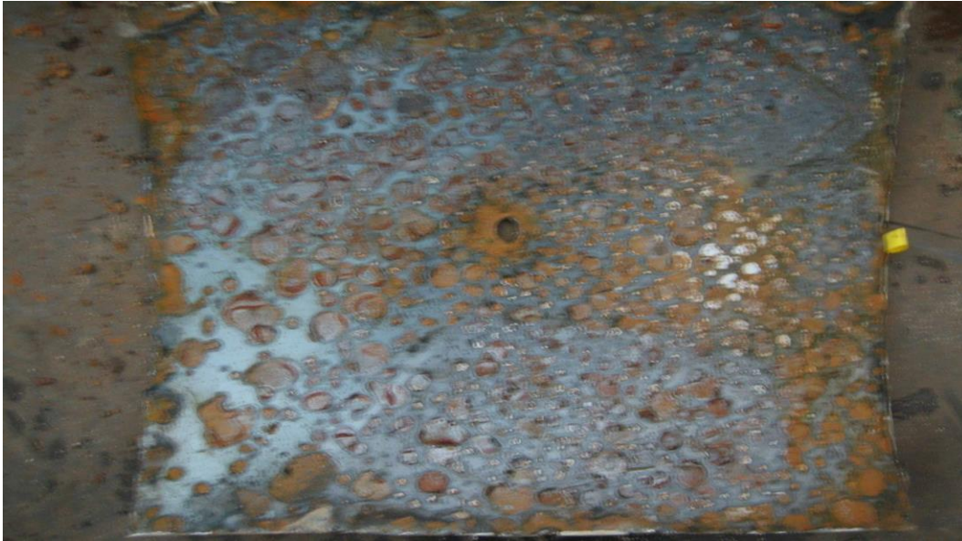
Figure 3.23. A sample of straight portion in a 700-mm diameter steel WTM before sandblasting for pipe cleaning
