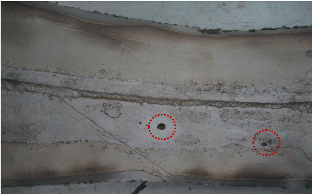
Figure 3.26. A pipe joint in a 900-mm diameter steel WTM after sandblasting for pipe cleaning, in which a few holes due to corrosion occurred on the joint weld and went through a pipe wall
