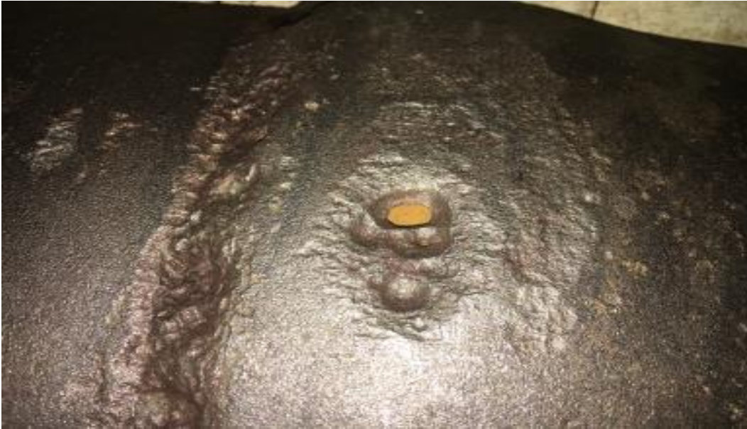
Figure 3.16. A hole due to corrosion around the weld caused a pipe break in a 350-mm diameter steel WTM.
