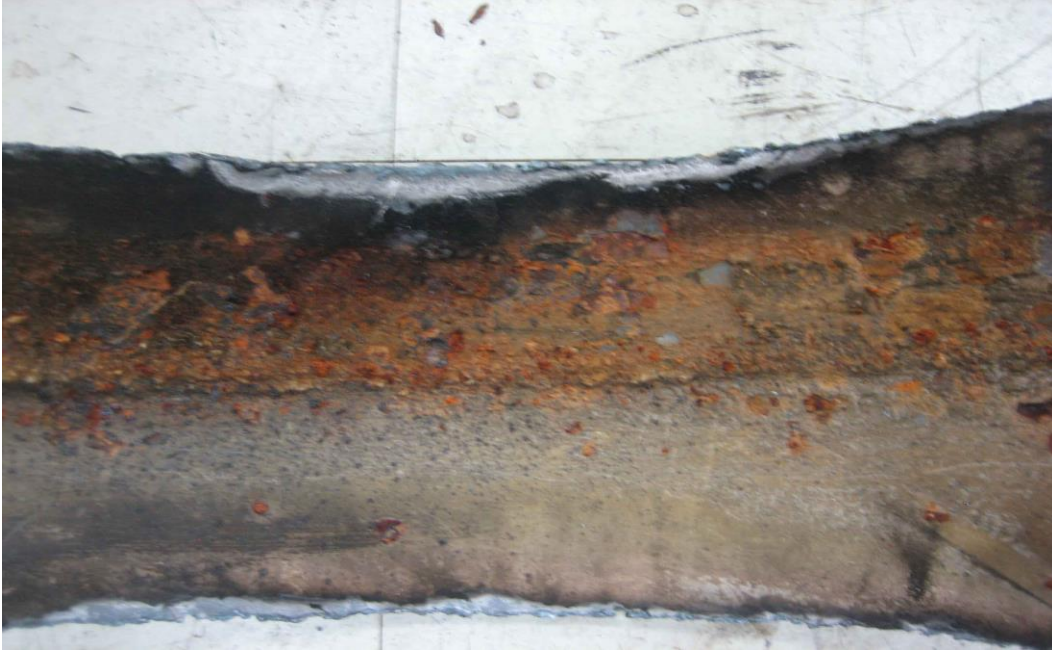
Figure 3.25. A joint weld in a 900-mm diameter steel WTM before sandblasting for pipe cleaning
