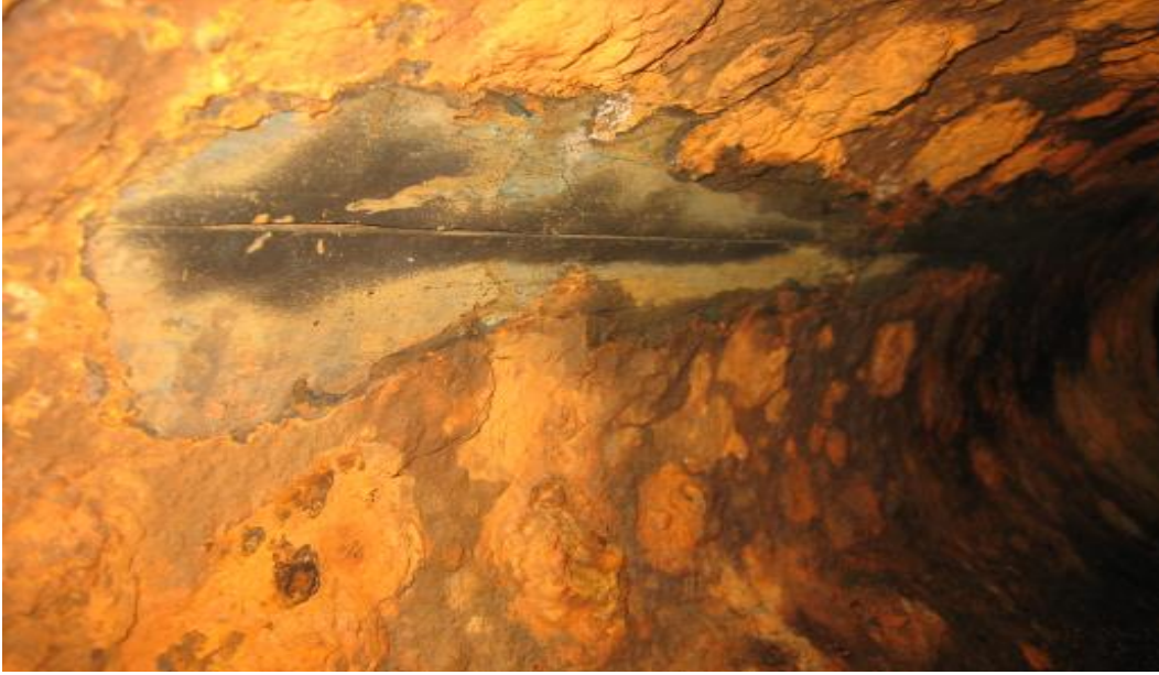
Figure 3.15. Corrosion forming around the longitudinal weld caused a pipe break in a 1,350-mm diameter steel WTM. Numerous tubercles and thick scales were built up.
