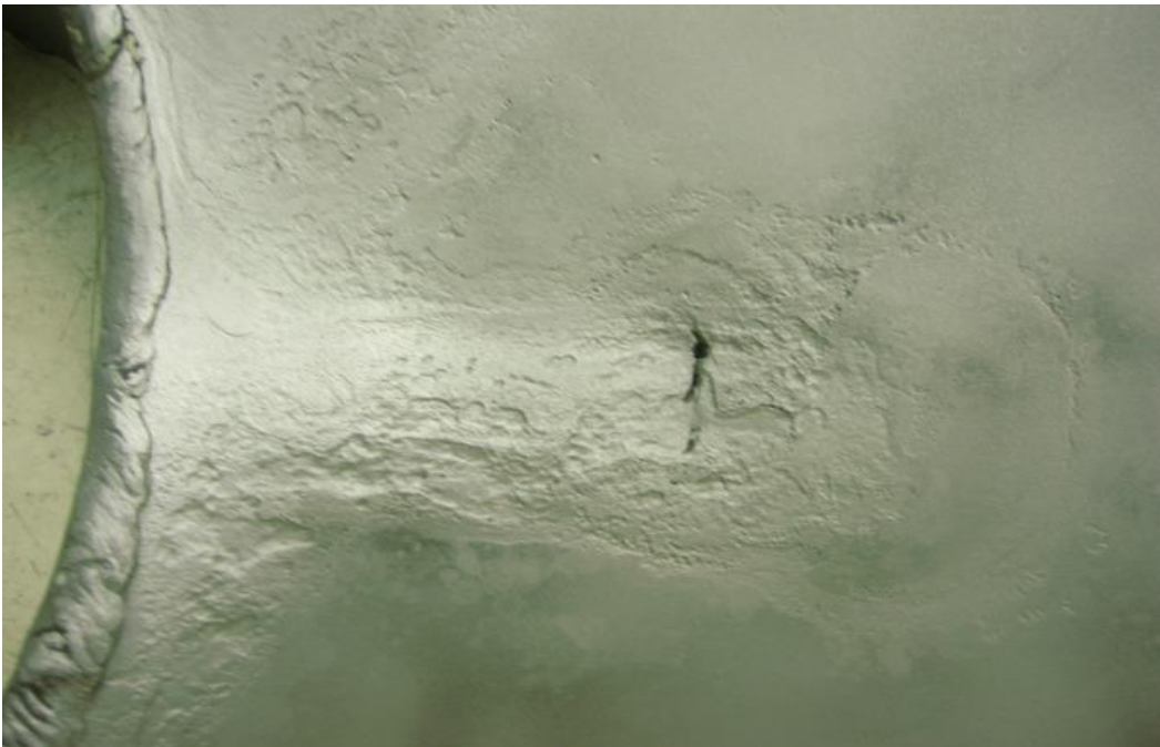
Figure 3.18. Appearance inside a 900-mm diameter steel WTM after sandblasting for pipe cleaning, in which the hole developed by corrosion caused a pipe break
