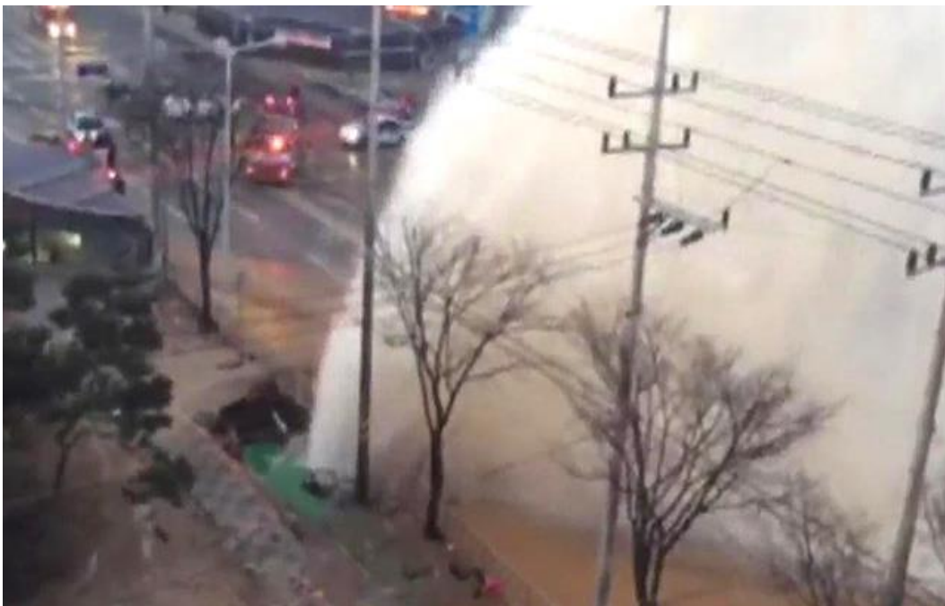
Figure 3.28. Broken water main floods homes, roads and cars in Pyungtack City in 2015 [source from (SBS NEWS 2015)]
