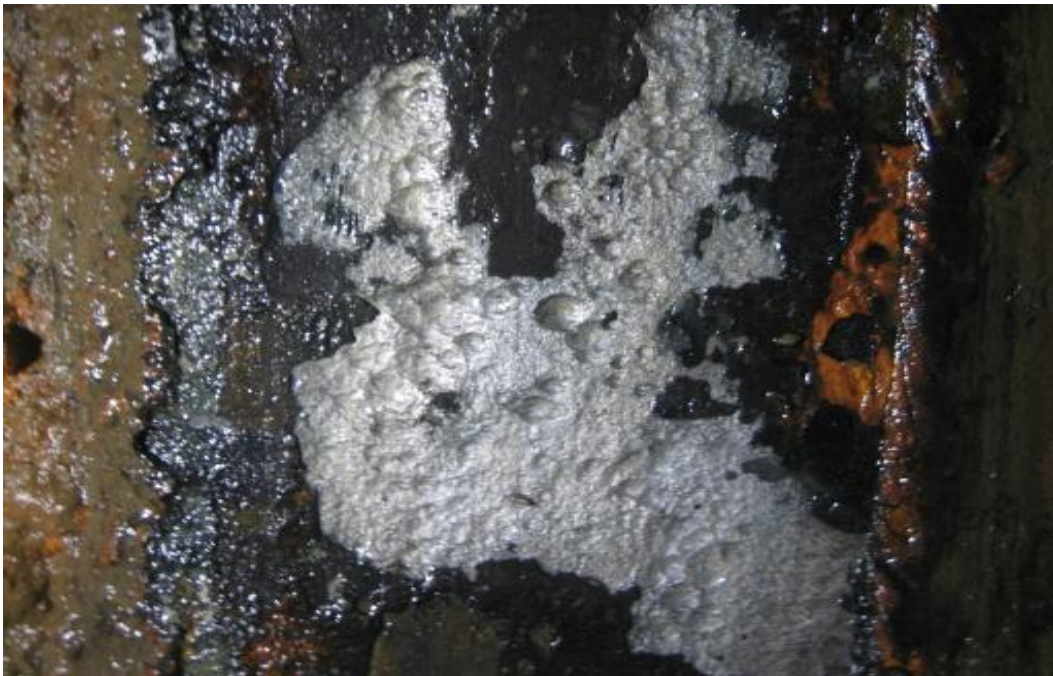
Figure 3.12. Corrosion developing inside a 1,650-mm diameter steel WTM.
