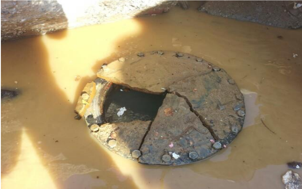
Figure 3.27. A crack on the pipe hole cover in a 2,000-mm diameter steel WTM, which was caused by temperature expansion and constriction, resulted in a flood in Pyungtack City, the ROK, in 2015.
