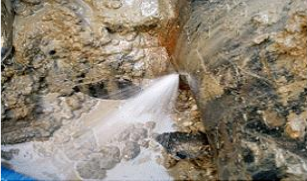
Figure 3.17. A pipeline leak in a 900-mm diameter steel WTM before sandblasting for pipe cleaning
