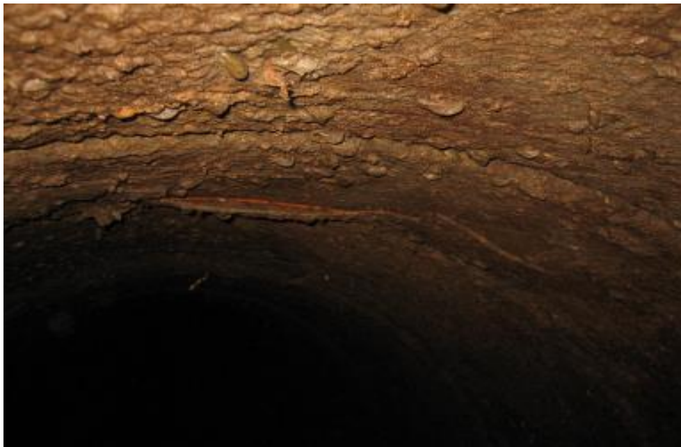
Figure 3.10. The internal coating material was cracked and detached at a pipe joint. The slime was developing across the 1,650-mm diameter steel WTM.
