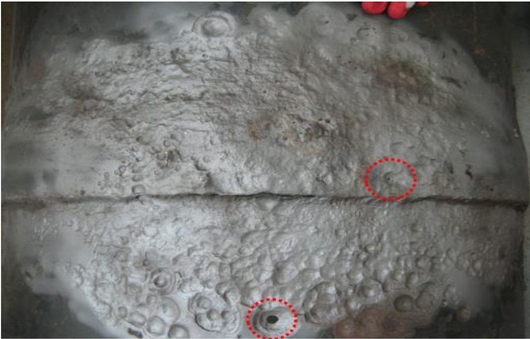
Figure 3.22. A 700-mm diameter steel WTM after sandblasting for pipe cleaning, in which numerous holes due to corrosion around a pipe joint weld caused a pipe break
