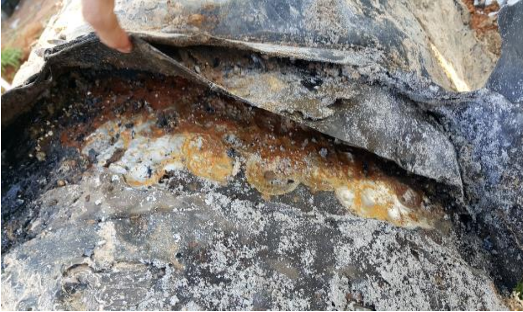
Figure 3.21. Appearance outside a 700-mm diameter steel WTM before sandblasting for pipe cleaning
