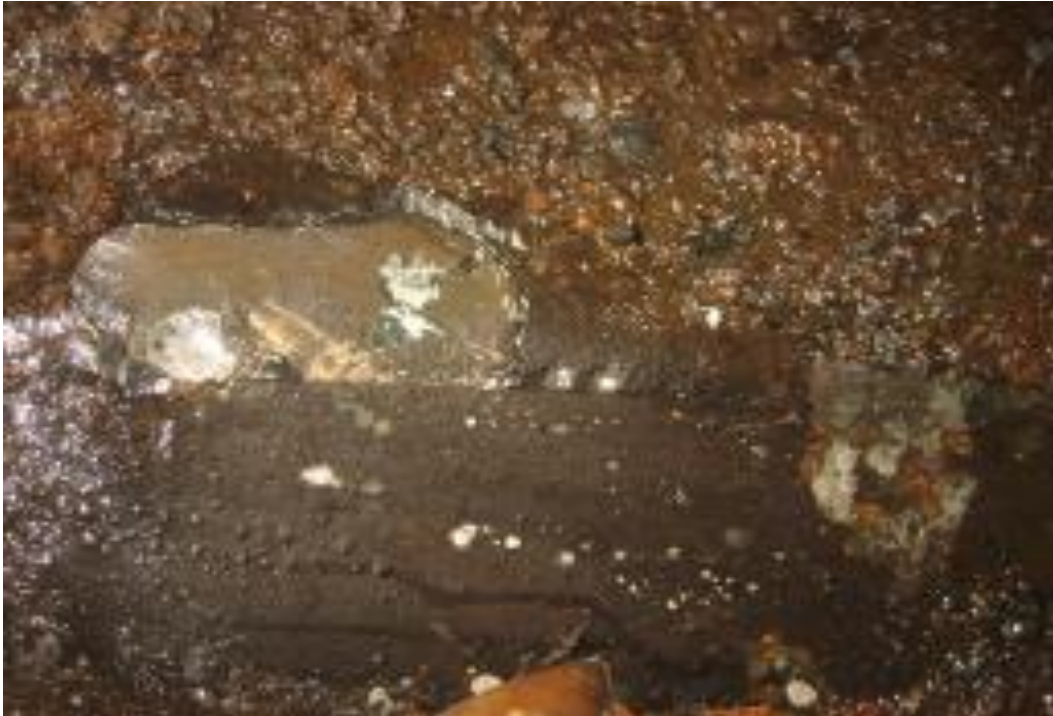
Figure 3.11. Corrosion developing at a pipe joint of a 1,650-mm diameter steel WTM.
