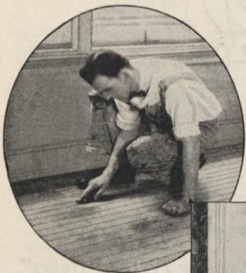
1 Left—A floor of well-nigh table-top smoothness is assured from the start. Two skilled workmen remove floor moulding and see that all boards are tight and even.
